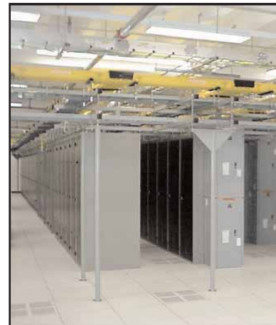
Atlanta 1 Colocation Area
