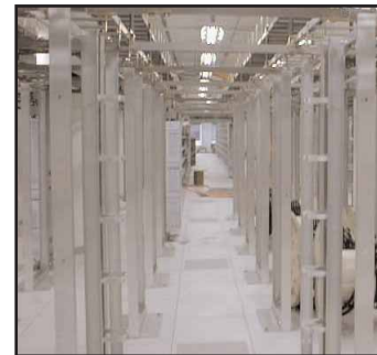
Chicago Colocation Area (North Canal Street)
