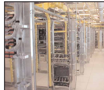
Cincinnati Colocation Area
