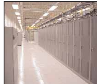
Dallas Colocation Area
