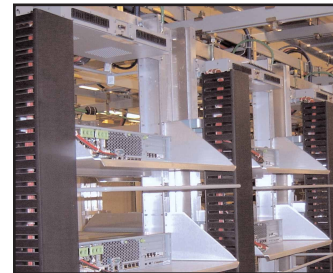
Denver Colocation Area
