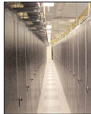
New York 1 Colocation Area
