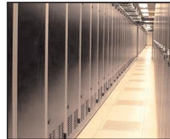
Philadelphia Colocation Area
