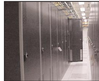
San Diego Colocation Area
