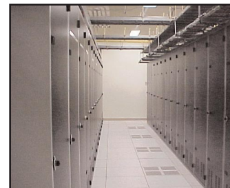
Stamford Colocation Area
