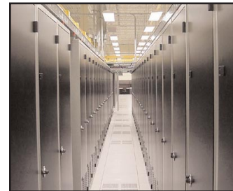
Tampa Colocation Area
